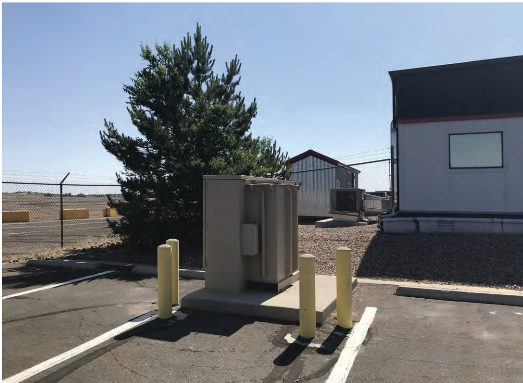
Image 2: Training center electrical transformer
